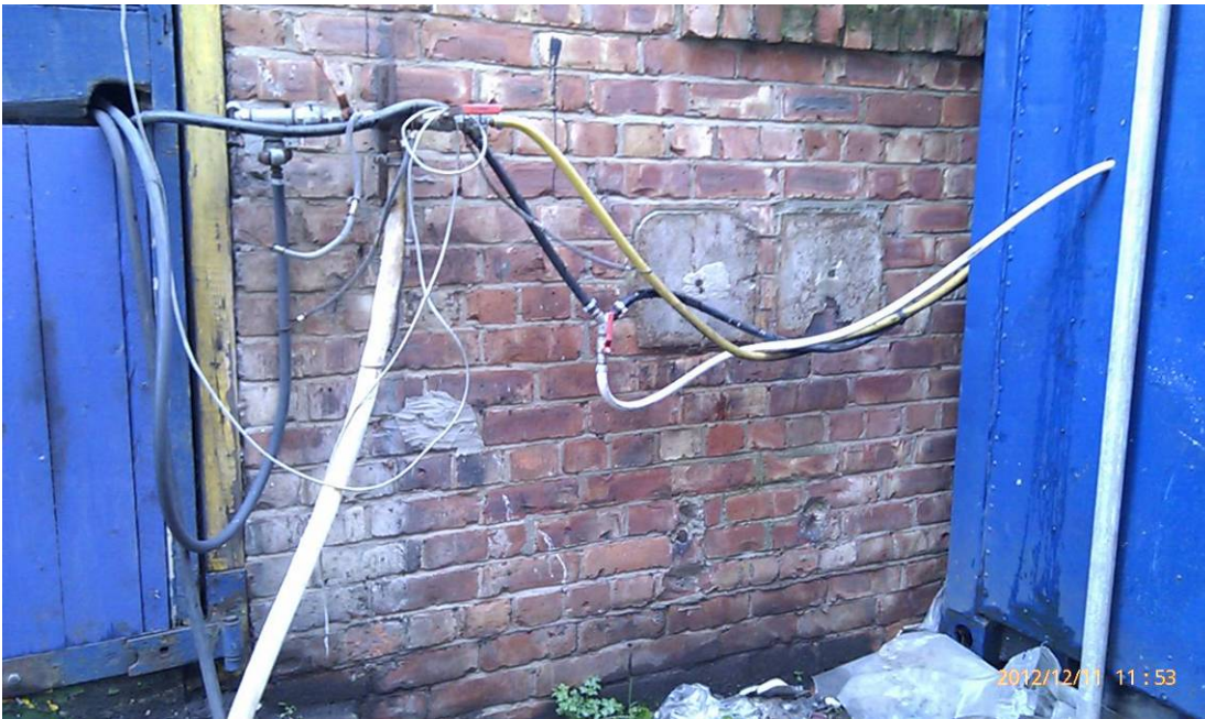
Water & Compressed Air Lines Feeding Portable Building Annex & Outside Discharge Valves
