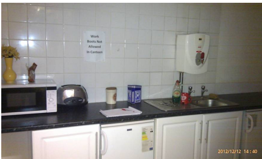
Kitchen. Electric Water Heater
