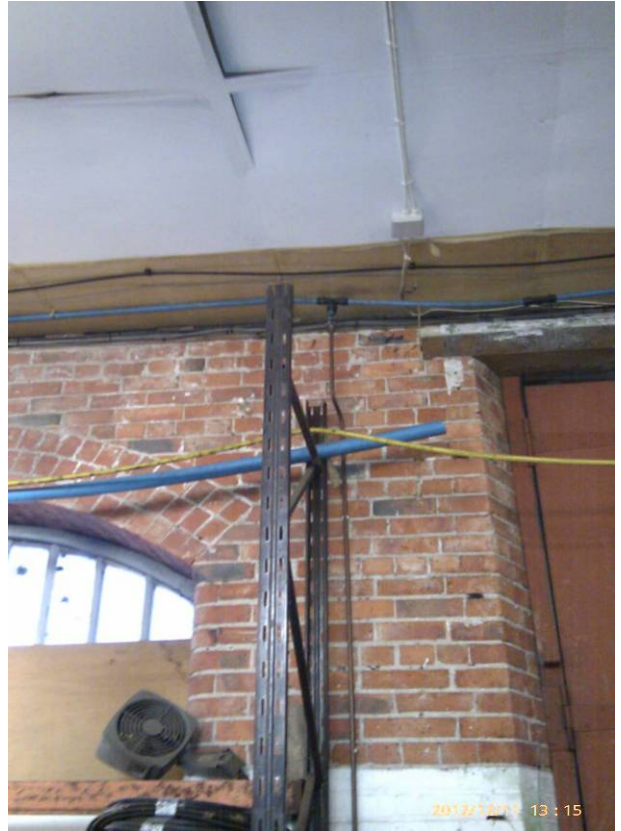
MDPE Water Services Distribution
