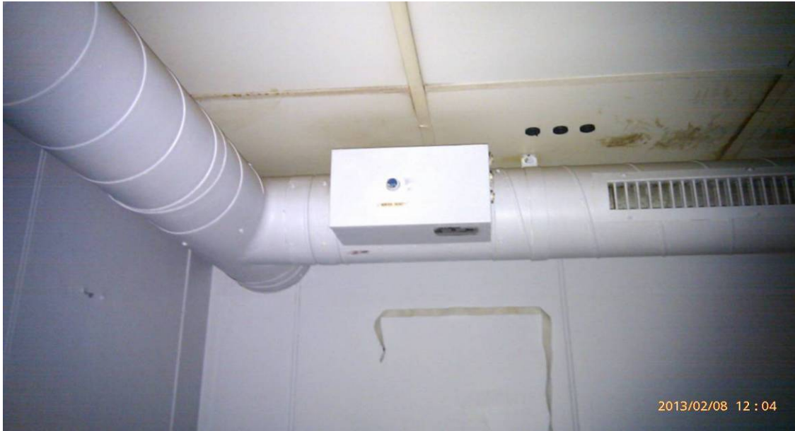
Redundant Duct Heating System
