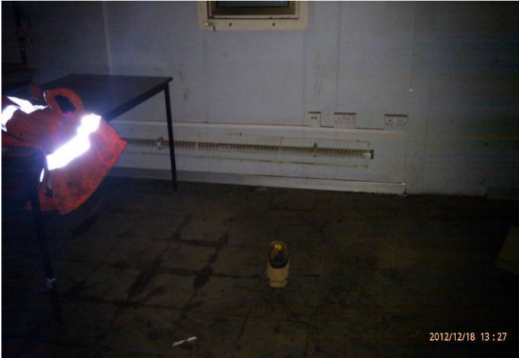
Electric Heaters Mess Area
