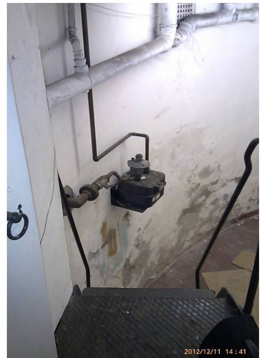
Offices (South) Gas Meter
