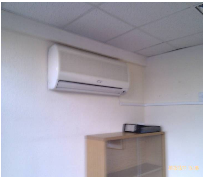
AC Unit. Conference Room
