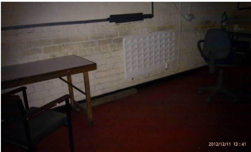
Pipe Shop Mess. Electric Heater
