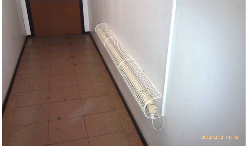
1 st Floor Offices, Corridor Electric Tubular Heater
