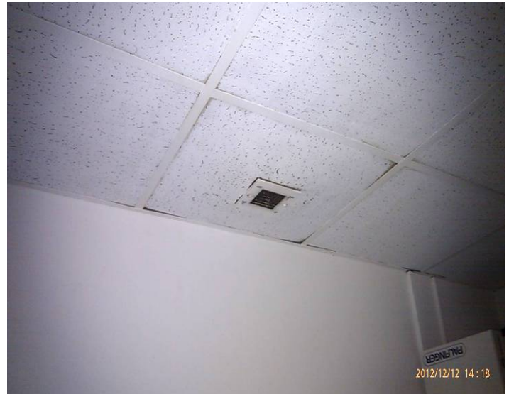
1 st Floor Offices, Corridor Ventilation Grille
