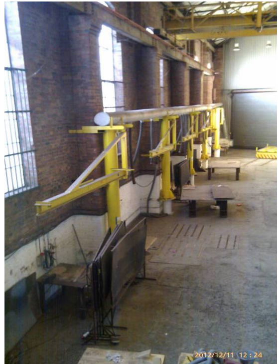
Main Pipe Shop. Specialist Extract Vent.
