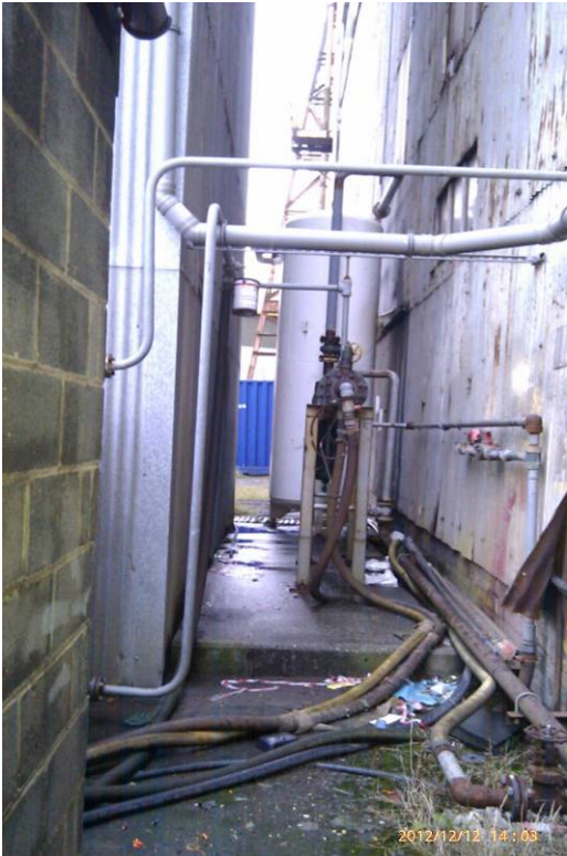
Comp Air Plant
