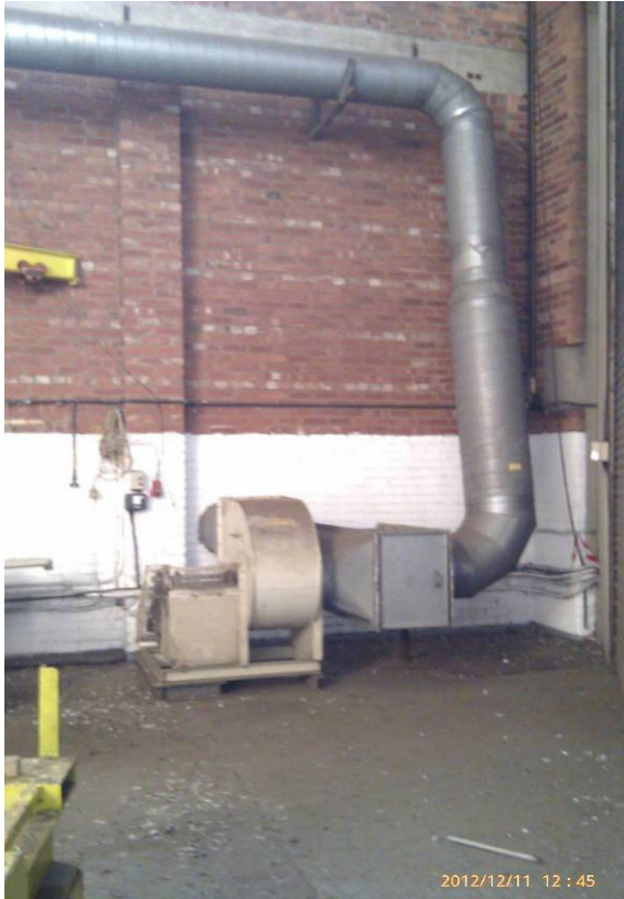
Main Pipe Shop Specialist Exhaust Ventilation System
