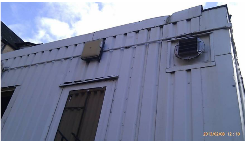
External Vent Duct
