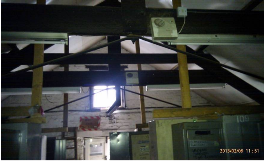
Locker Room Electric Fans
