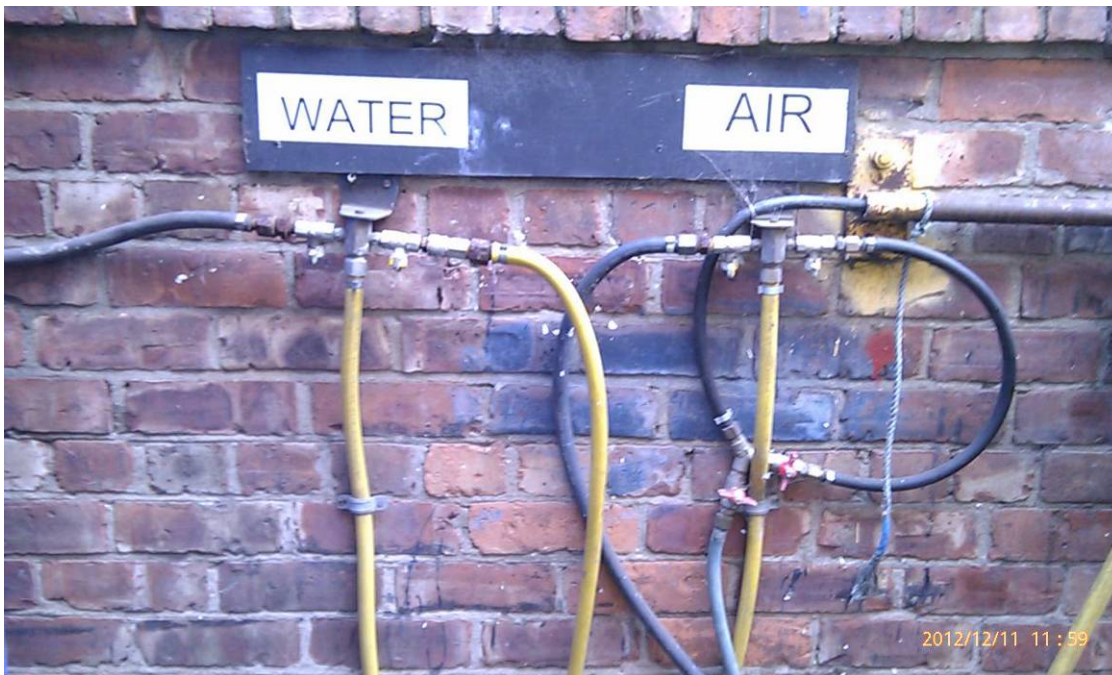
Water & Compressed Air Lines
