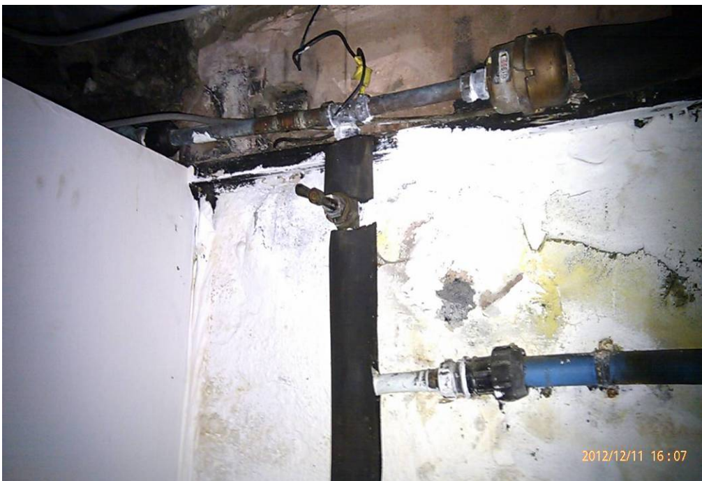
Water Meter (Basement)
