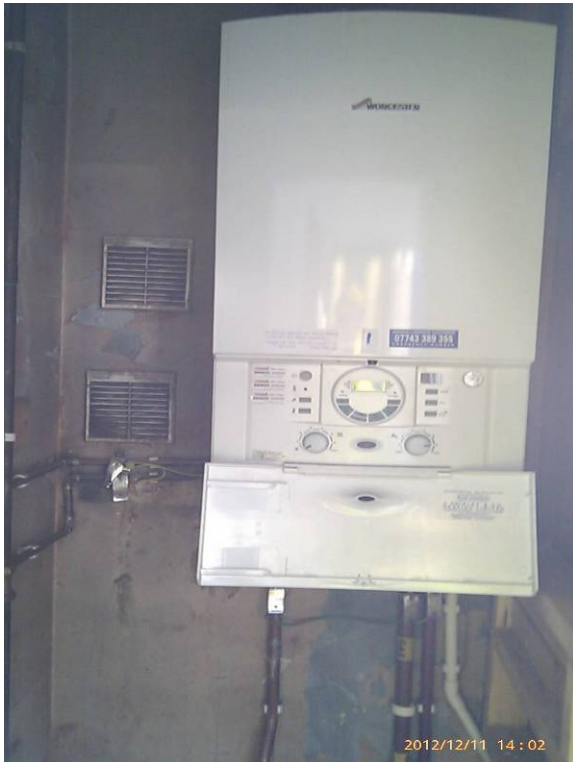
Offices LPHW Boiler
