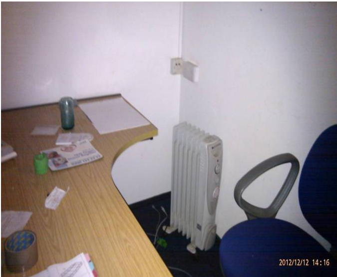
1 st Floor Offices, Corridor Electric Heater
