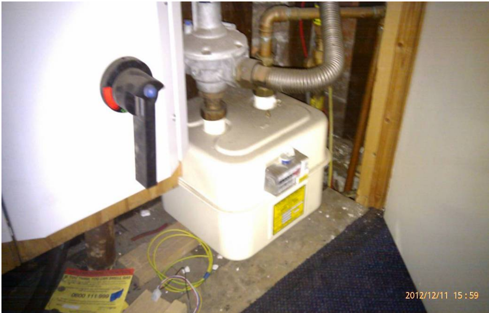
Gas Meter (Ground Floor Lobby)
