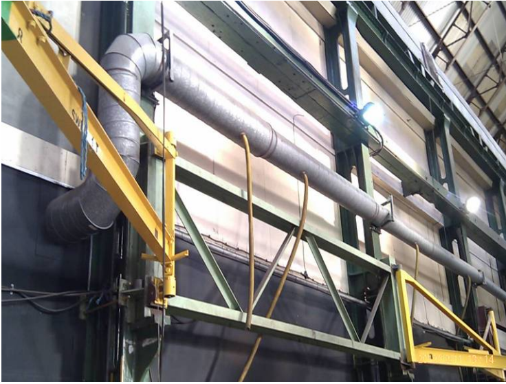
Welding Specialist Ventilation System
