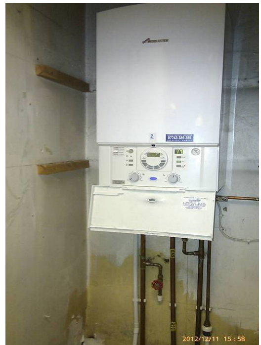
Combi Gas Boiler located in cupboard on stair landing
