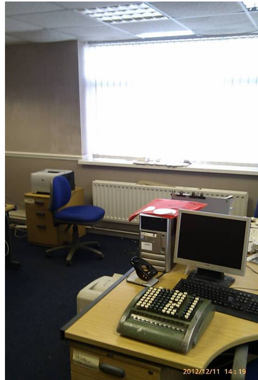
LPHW Heating in Offices (South)
