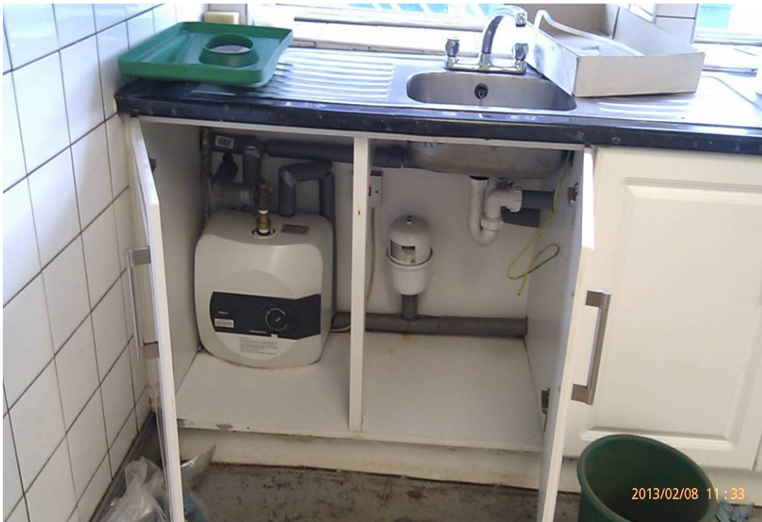
Mess/Kitchen Electric Water Heater
