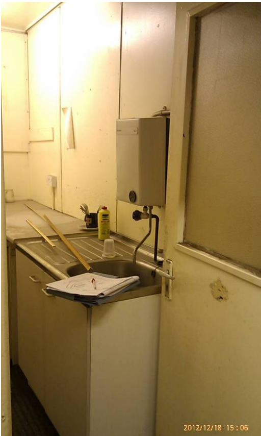
Electric Water Heater
